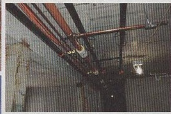
North Central College's combo dorm-field house utilizes a radiant floor heating system.
